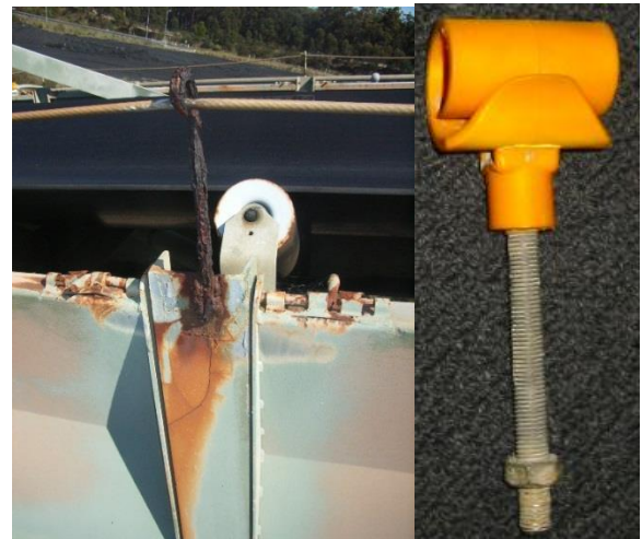
Figure 4: Alternate materials to solve an OHS corrosion issue
