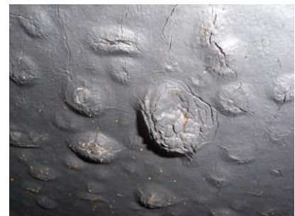
Figure 2: Premature coating failure due to inappropriate coating specification & poor application methods
