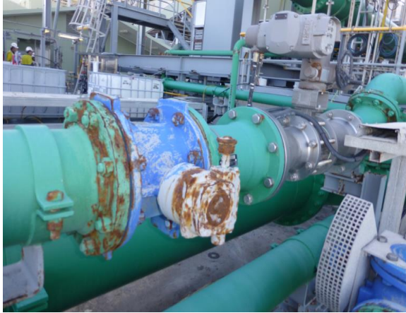
Figure 3 – Dissimilar metals in direct contact; causing accelerated corrosion damage to the less corrosion resistant alloy.
